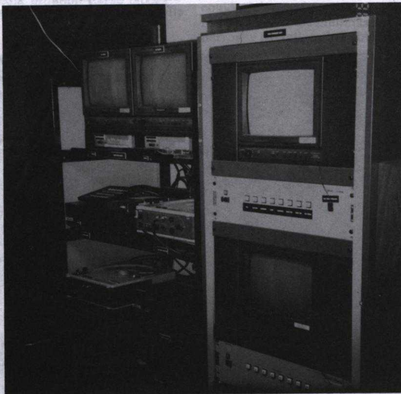
Fig. 2. The control room for the high-tech classrooms.
