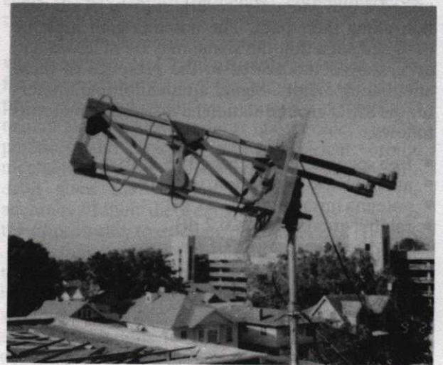
Fig. 4. Roof-mounted VHF antenna.
